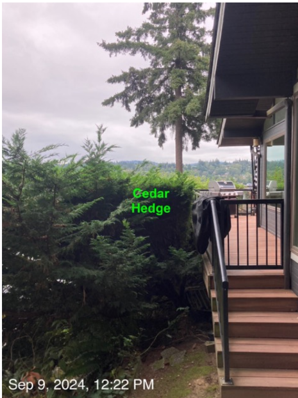
Cedar portion of hedge on N property line noted as overgrown on sides. Cutting back may leave trees non-viable. Eventual removal and replacement with more site appropriate species.
