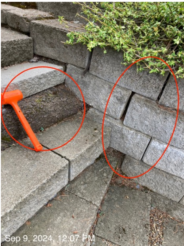
Significant damage from tree #1 to adjacent block retaining wall. Cutting of the offending root would leave the tree non-viable and non-wind firm.
