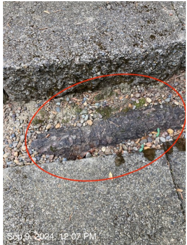
Large exposed roots would need to be cut to repair stairs, leaving tree #1 non-viable and non-wind firm.
