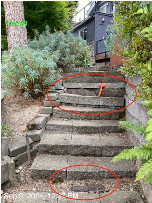
Subject tree #1 has caused significant damage to stairs and wall to NW due to soil displacement from root growth.
